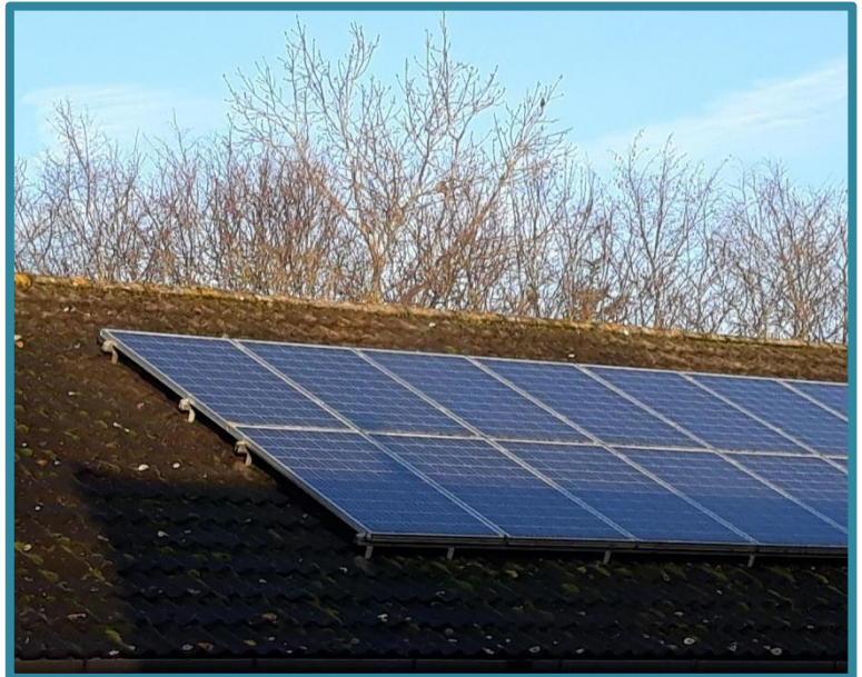
Solar panel shading
